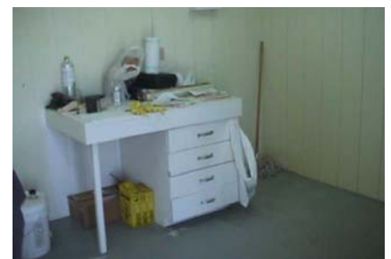
Water monitoring equipment in Well House
