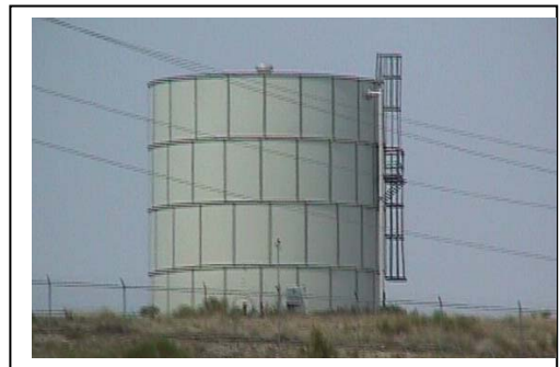
Water Storage Tank North of Burlington
